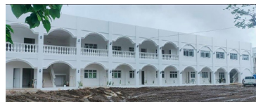
CONSTRUCTION OF 2-STOREY CIES ACADEMIC AND LABORATORY BUILDING AT CSU GONZAGA Percentage Completed: 100%
