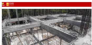
CONSTRUCTION OF 2-STOREY ACADEMIC AND LABORATORY BUILDING AT CSU LASAM Percentage Completed: 56%
